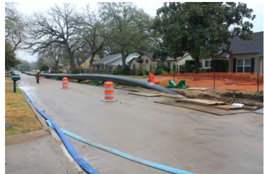
Residential area with limited ROW and mature landscaping. 30-inch HDPE pipe enters insertion
